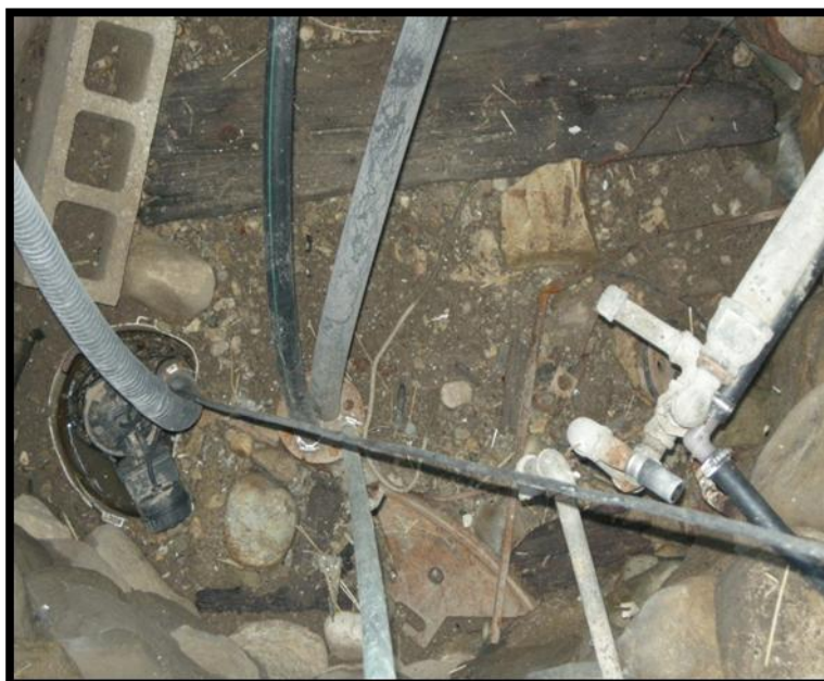
Figure 4: Poorly maintained wells can provide a conduit for contaminants to travel from the surface down to the aquifer. (SGSNBP Source Protection Region)
