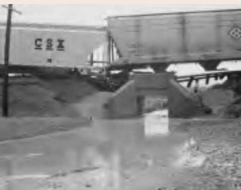
Erosion damage to rail line
