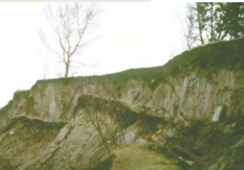
Slumping of slope on Lake Huron shoreline
