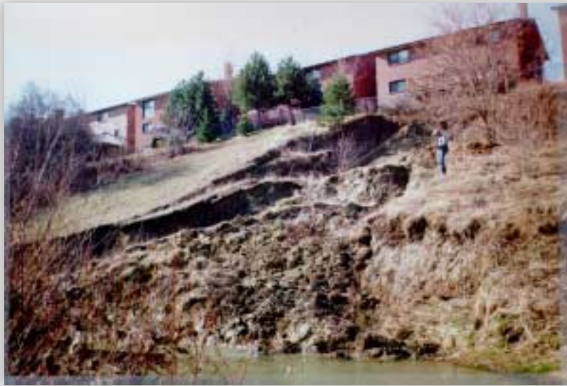
Figure 1 - Slope Slide Caused By River Erosion
