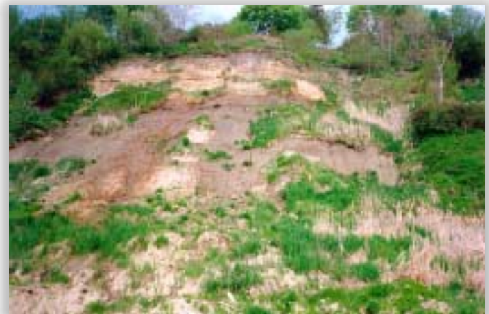
Figure 82 - Scarps, Slumped Soil Masses
